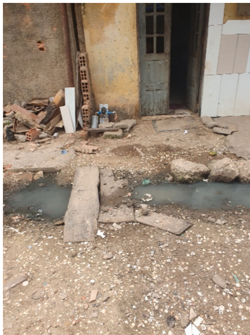
Fig. 2. Wastewater in the streets of Barra de Santo Antônio, Alagoas. Source: Photo taken by the first author, 2025.
