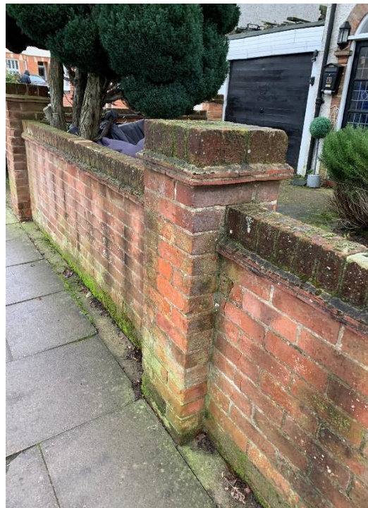
A low half brick boundary wall with brick and half end terminal and intermediate piers.
