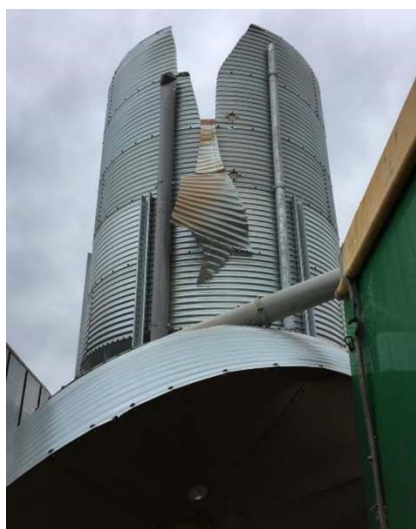
Figure 14 Silo With Top Blown Off Due to Over-Pressurisation. The Top Cone and Ring of the Silo Are Lying in the Bottom of the Picture
