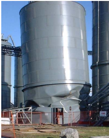
Figure 16 Steel silo with buckled unstiffened skirt
