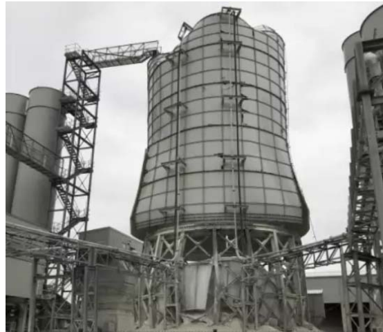
Figure 7 Failed Silo Constructed From Flanged Panels
